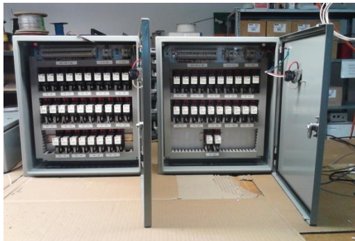
Voltage monitoring heat trace panels
